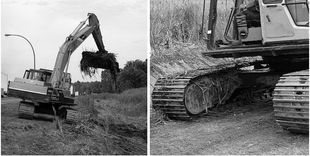
FIGURE 7. An excavator working along a highway in southwestern Quebec, where it is being used to deepen a roadside ditch. The excavated substrate containing rhizomes of Phragmites australis subsp. australis will be transported to a landfill, and rhizomes with shoots can be seen lodged in the tracks. The vehicle will likely introduce rhizomes to the next work site. Photo by P.M. Catling in southwestern Quebec in 2005.
